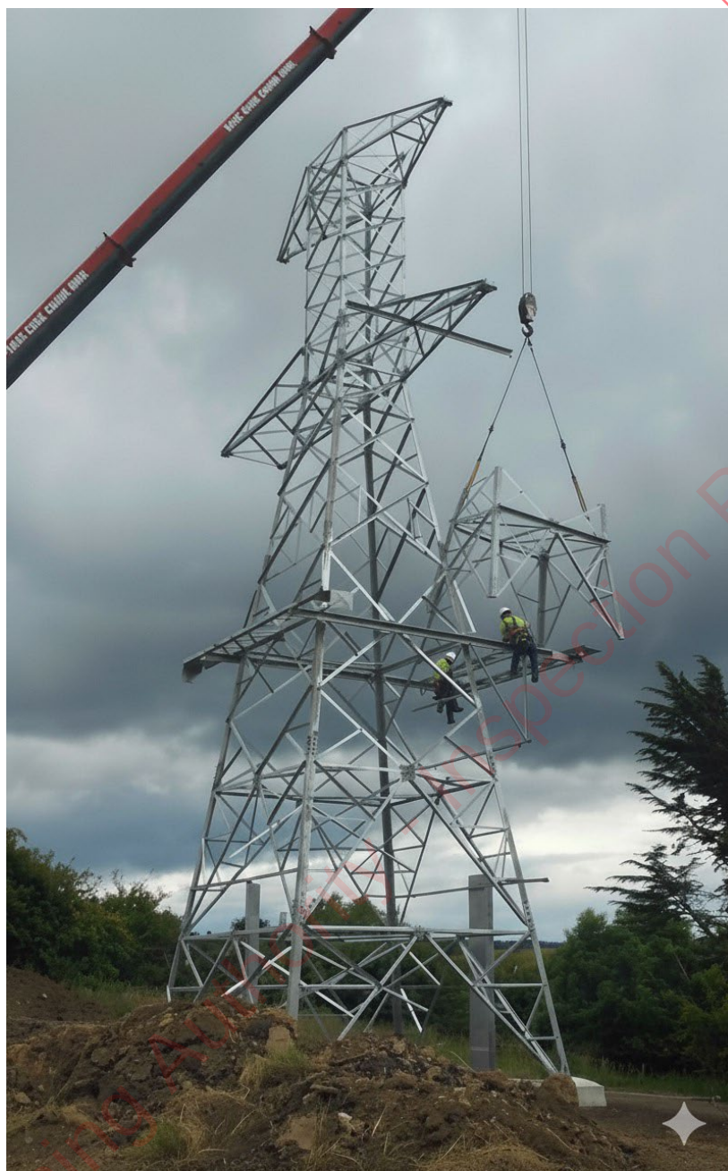
Figure 5: Cable End Mast
