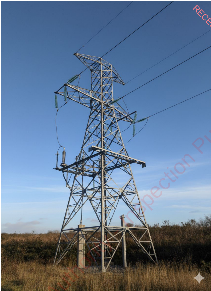
Figure 6: Cable End Mast
