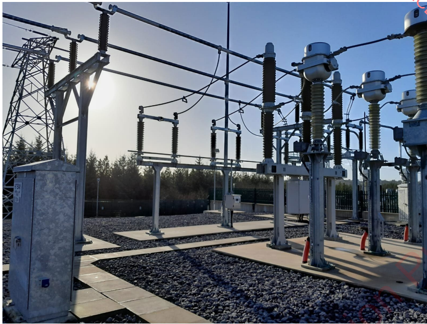
Figure 7: Typical 110kV Electrical Infrastructure
